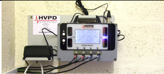
The HVPD Mini™ Monitor installed on its wall mounting bracket in a substation
